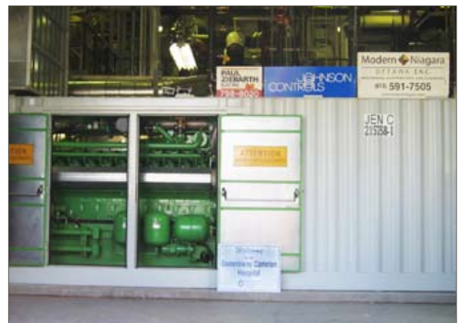
The Jenbacher system at Queensway-Carleton Hospital.
