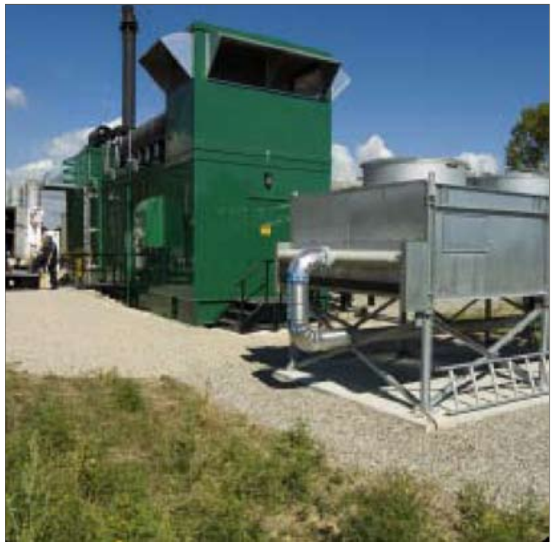
The Woodward Avenue waste water treatment plant is now a valuable source of renewable energy thanks to a biogas CHP system.
