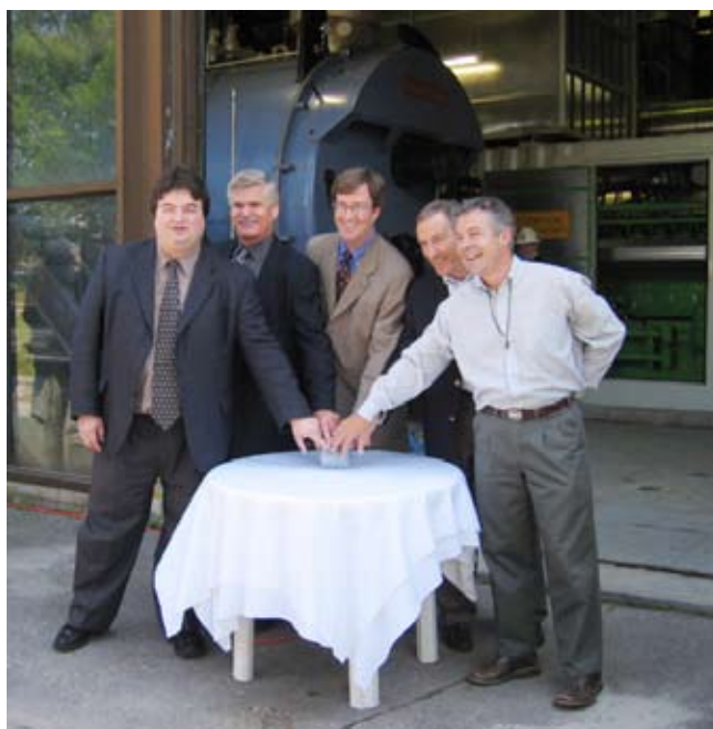
Firing up the combined heat and power system at Queensway-Carleton Hospital. The system saves the hospital $350,000 per year in utility costs.
