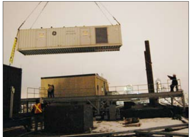
A combined heat and power system was recently installed on the roof of Toronto Housing's David A. Croll apartments.
