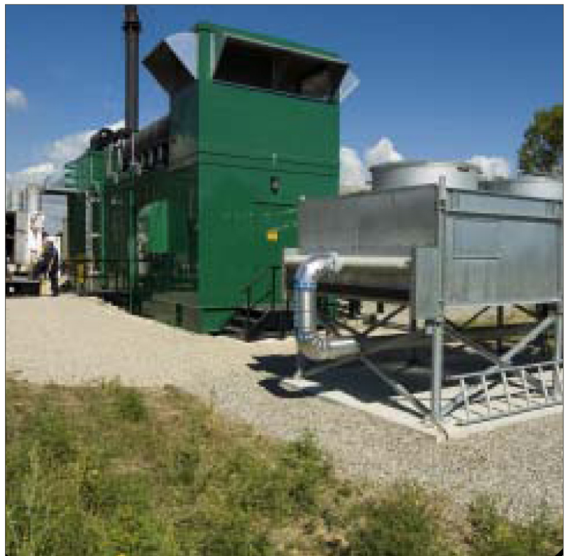
The Woodward Avenue waste water treatment plant is now a valuable source of renewable energy thanks to a biogas CHP system.
