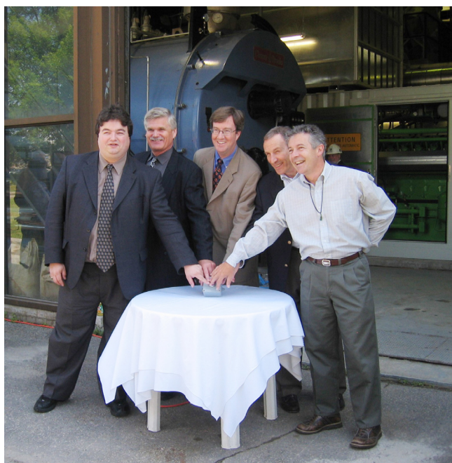
Firing up the combined heat and power system at Queensway-Carleton Hospital. The system saves the hospital $350,000 per year in utility costs.
