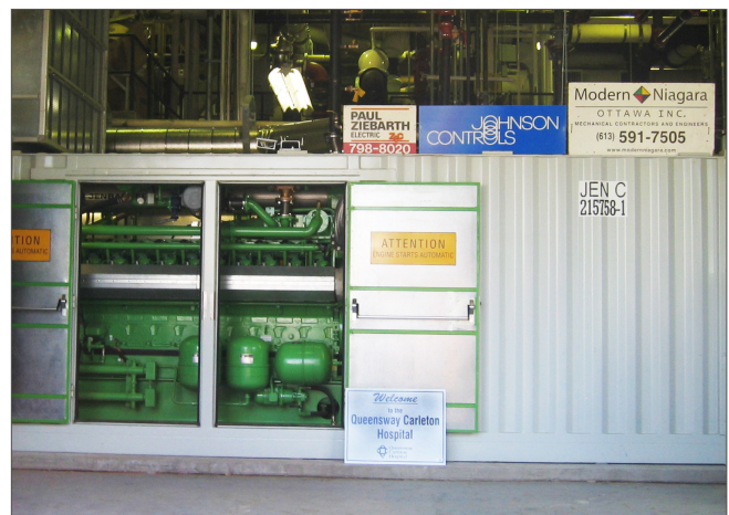
The Jenbacher system at Queensway-Carleton Hospital.
