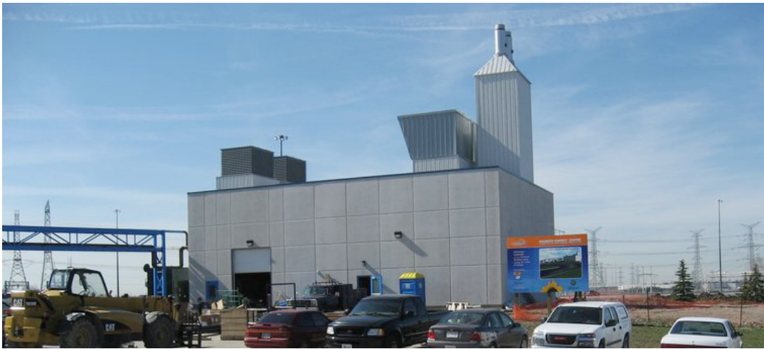
The Markham District Energy System will have four locations when completed. Photo left – Construction nears completion on the second site in April 2008.
